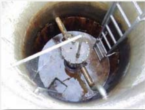
The leaking area
